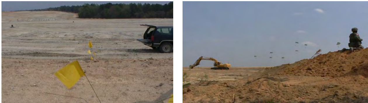
Figure C-5. Earth work including leveling, grading, and terrace construction at Holland DZ, Fort Bragg, NC.
