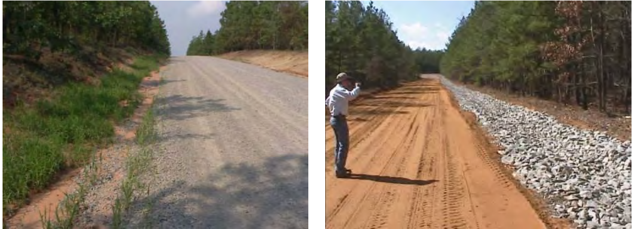
Figure F-2. Tank trail improvements to McKellers Road, Fort Bragg show Army CARES implementation that fits the particular topography, soils, and natural/native vegetation of the site.
