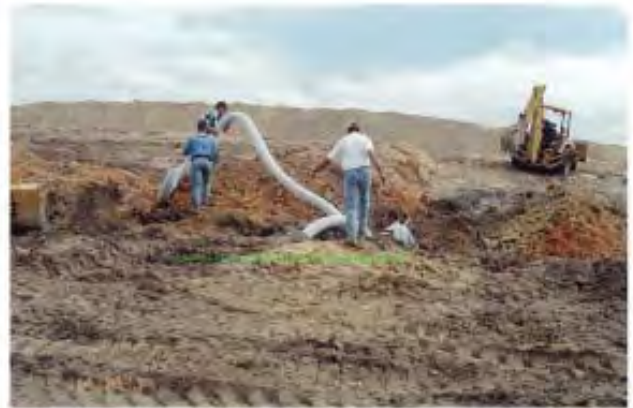
Figure C-8. Subsurface stormwater drainage system.
